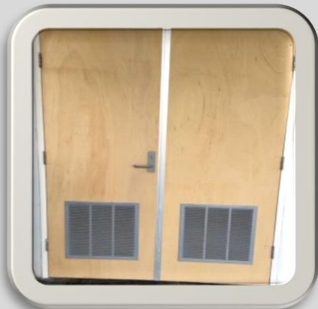
Fire Rated Doors with Air Grill
